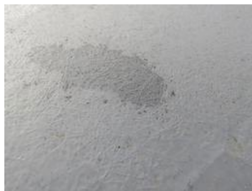
Visible fibre glass to rear flat roof
