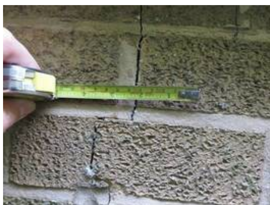
Cracking below window to North elevation
