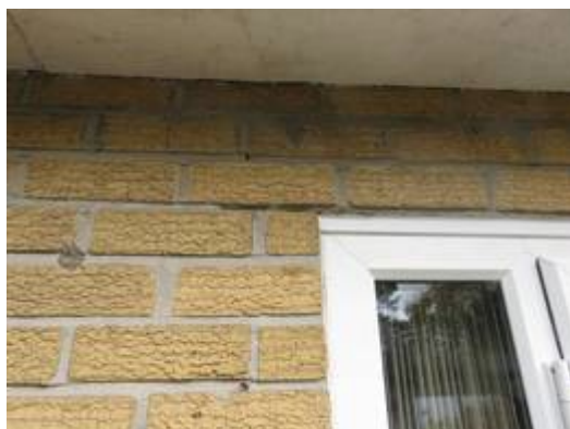
Minor corrosion to lintel above rear lounge external door
