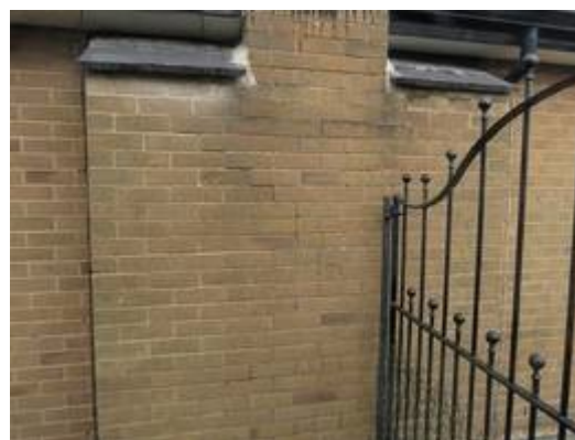
Cracking to chimney breast to South elevation
