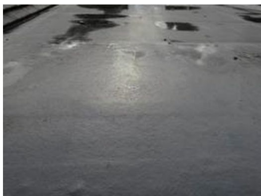
Visible fibre glass to rear flat roof
